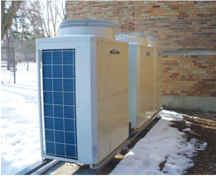
An ultra-high efficiency heating and cooling system is installed at the school district administration center.
